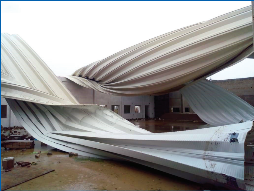
Roof of Om Shanti Auditorium, Godly Rajyoga Retreat Centre, Puri blown-off by cyclone 'Fani'.
