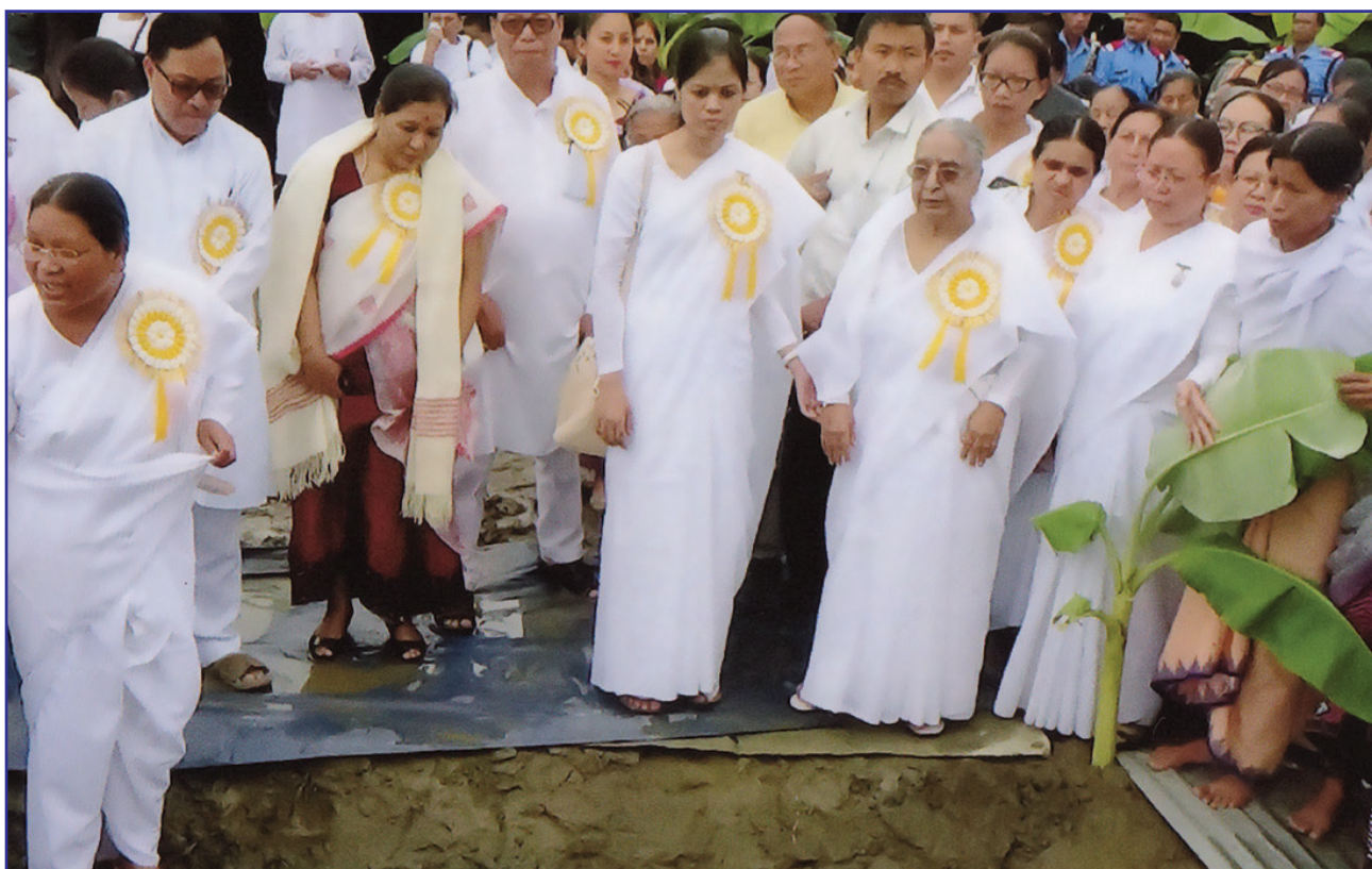
Imphal, Manipur: During the foundation laying of a new building, present are Dr. Ratan Kumar Singh, Hon'ble Minister of Education & Transport, Mrs. O. Landhoni, MLA, Mrs. W. Brajabidhu, MLA, BK Sheela, BK Nilima and others.
